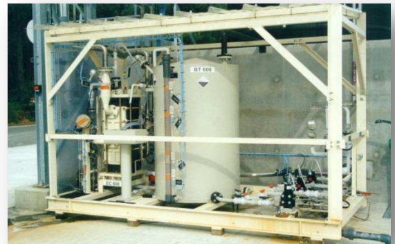
Skid assembly for 98% sulfuric acid dilution; yields acid that is diluted at 40%
